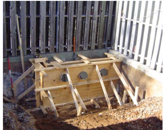
Field constructed concrete containment with oil stop valves
