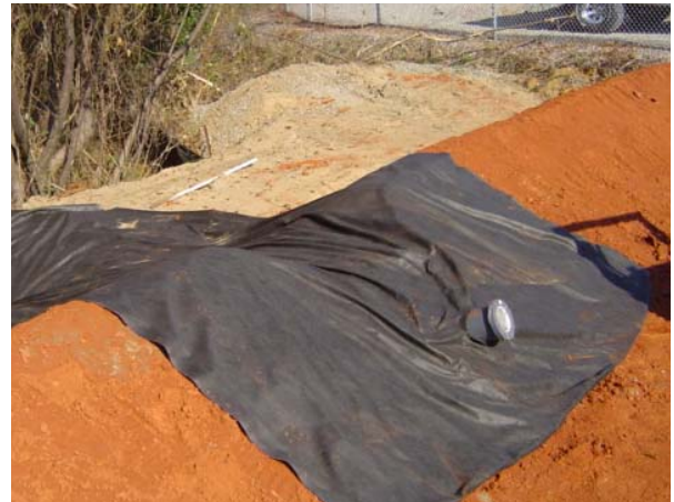
Oil stop valve in earthen berm
