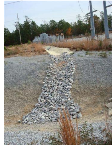
Lined channel to gravity oil / water separator
