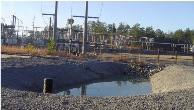
Gravity oil water separator (direct flow from substation)
