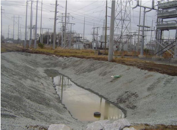
Gravity oil / water separator (pipe and channel inflow)
