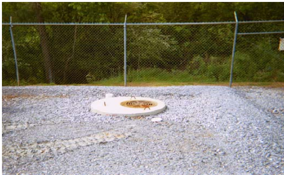
Catch basin with oil flow restrictor
